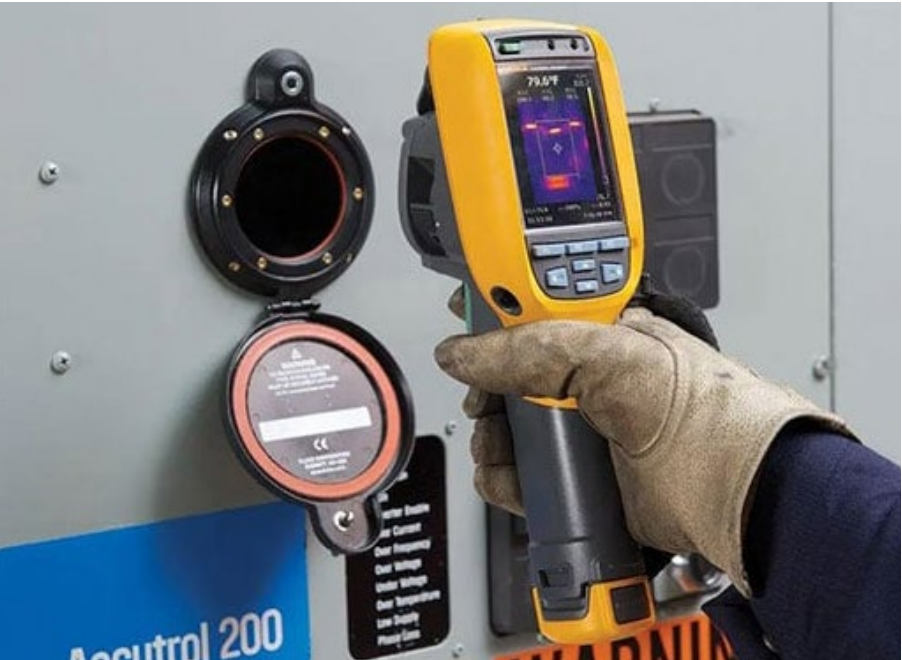
Figure 2: Shown is an example of an IR window mounted on a control panel, allowing access for a thermal imaging camera. Source: Fluke Electronics
