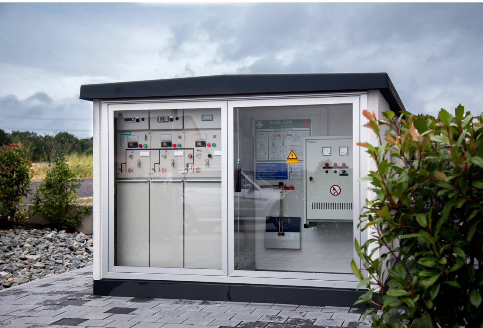
Substations as Nodes in the Distribution Grid
