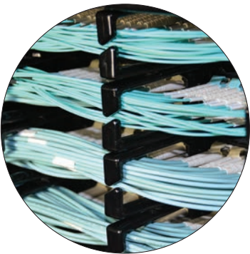
Front cable management
